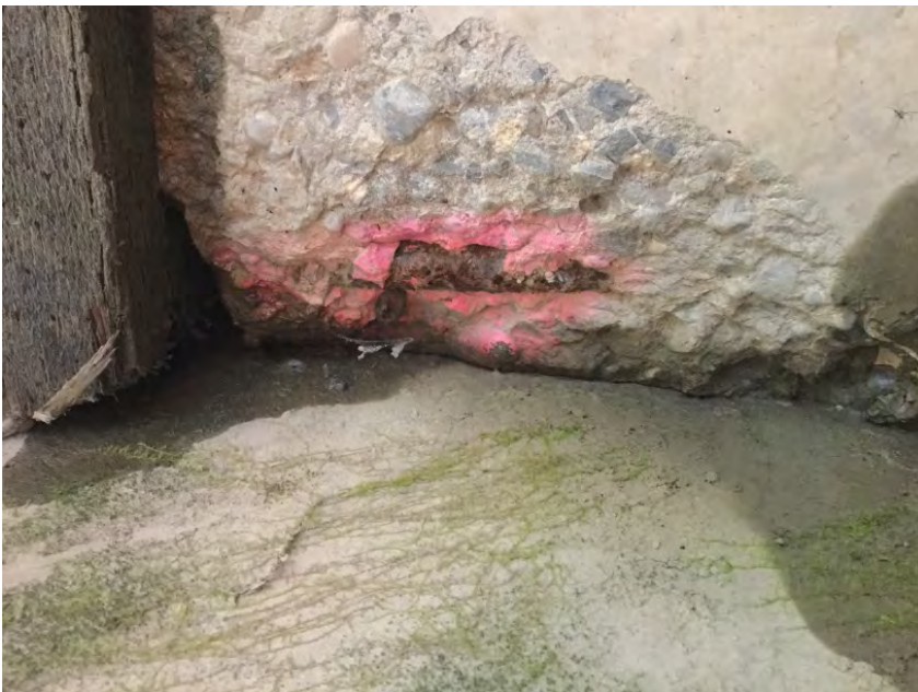
Deck panel damage with rebar exposed
