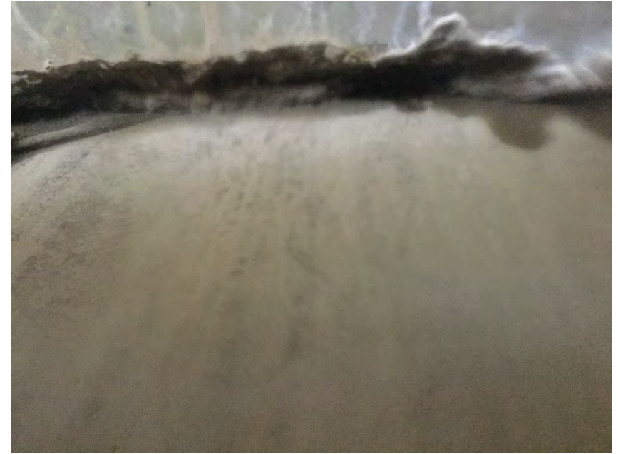
Deck panel damage
